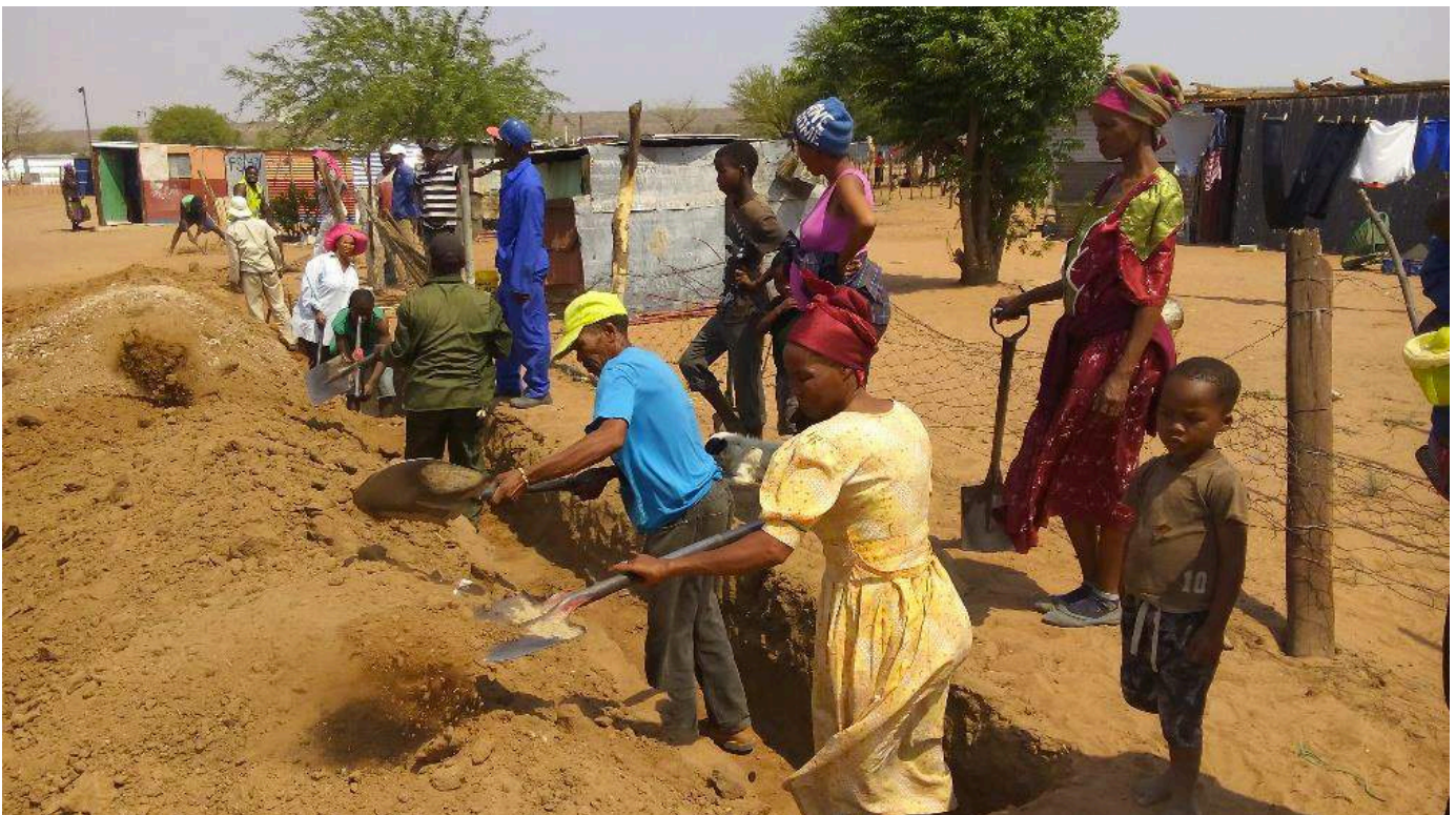
Freedom Square community participating in the digging of trenches for water pipes, with 44 people trained how to install water pipes for all 1030 plots
